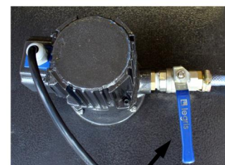
Pump valve closed
